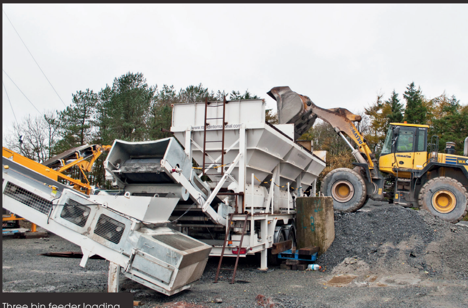
Three bin feeder loading
