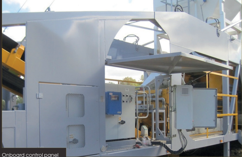
Onboard control panel
